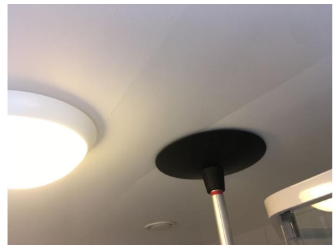
Sprekker i himlingsplater
