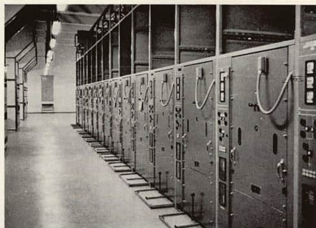
22 kV, koblingsanlegg for regulert spenning.
