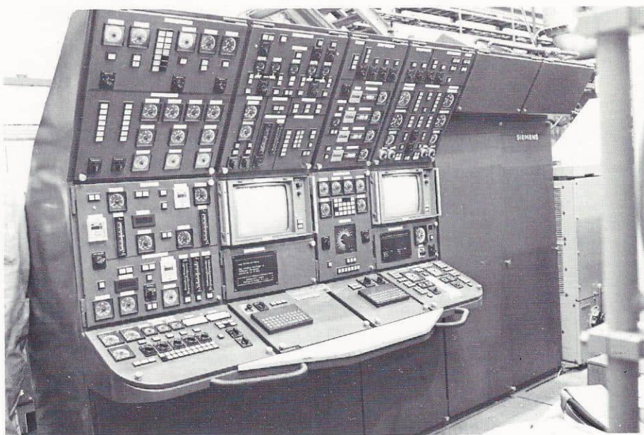
Engineering Control Console (ECC) – Siemens Bergen
